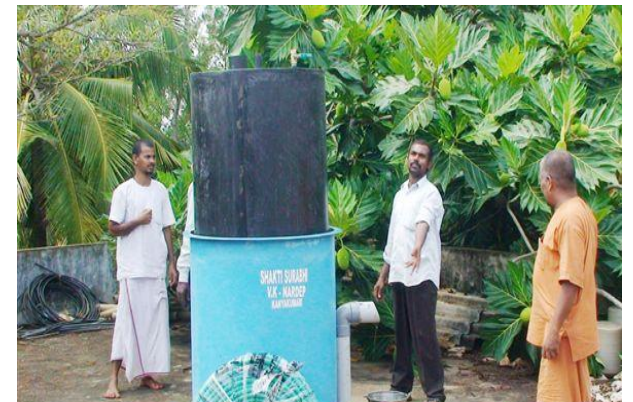
Commissioning of Shati Surabhi bio- methanation plant at Vivekananda Ashram, Vellimalai, Kanyakumari District.
